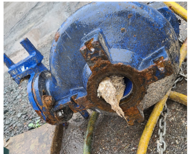
ASC pump clogged with "flushable wipes"
