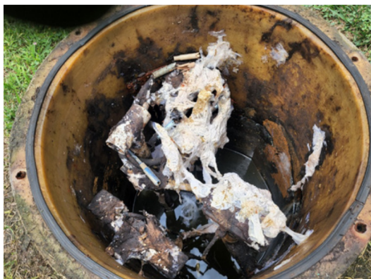
Disposable wipes clogged up in a sewer line grinder
